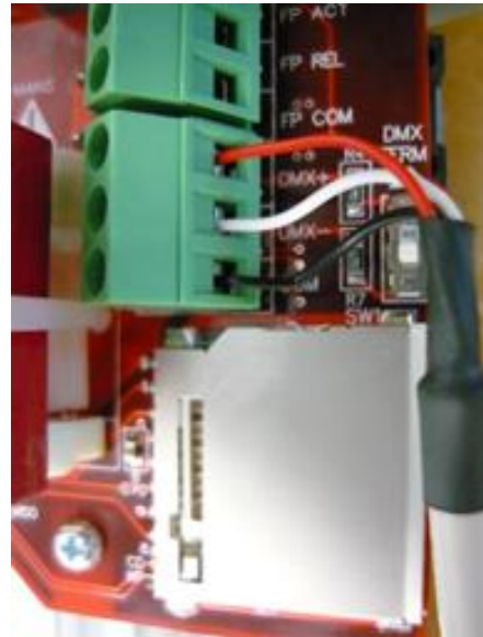
DMX cable connection detail
