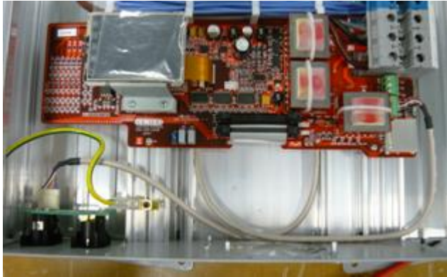
Internal wiring and cable routing. Left hand cover panel removed to show cable routing. Leave in place to avoid damage to static sensitive control electronics.
